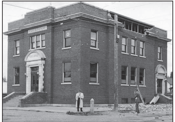
Courtenay B.C., masonry failure of post office
