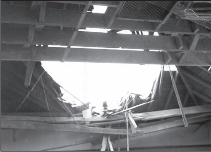
Courtenay B.C., chimney collapse through roof of elementary school
