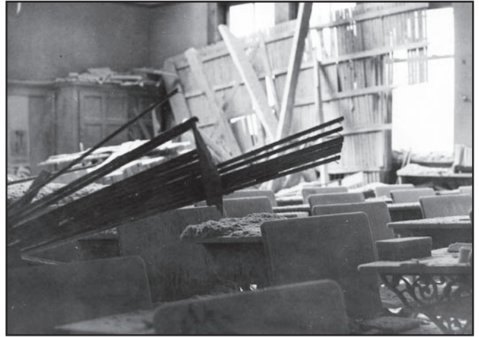
Courtenay B.C., damage to interior of elementary school
