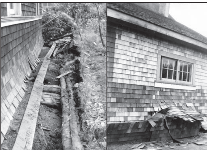
Comox B.C., earthquake damage and house foundation failure
