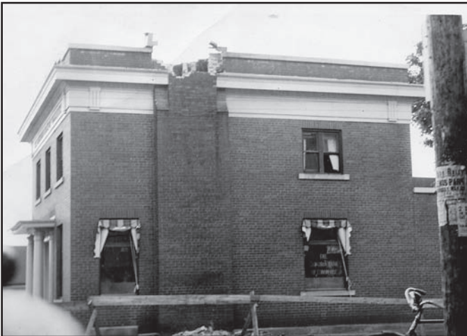
Courtenay B.C., damage to the Canadian Imperial Bank of Commerce
