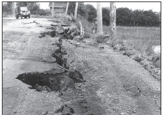
Comox B.C., earthquake damage on Comox Road
